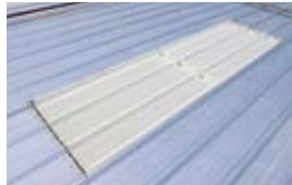
The roof features 26-gauge Galvalume® LibertyRib® panels and three translucent light panels that allow natural day light into the building.
